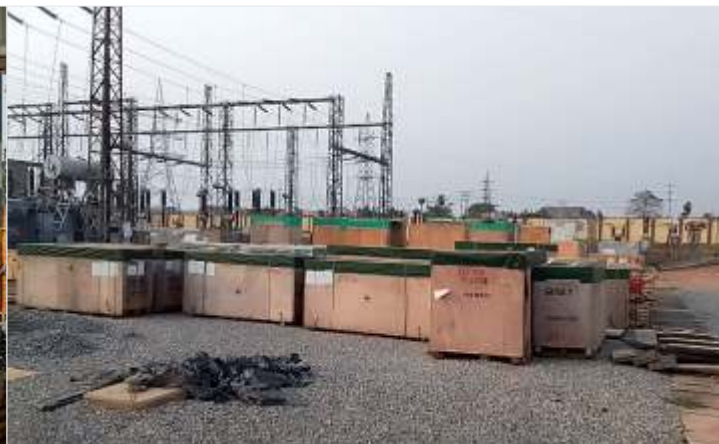
Transformer accessories in Ota 132/33kV Transmission Substation
