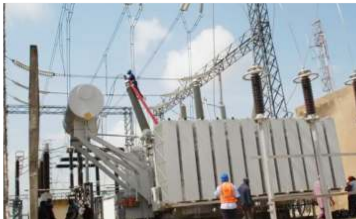
150MVA, 330/132kV power transformer energized at Ayede Transmission substation
