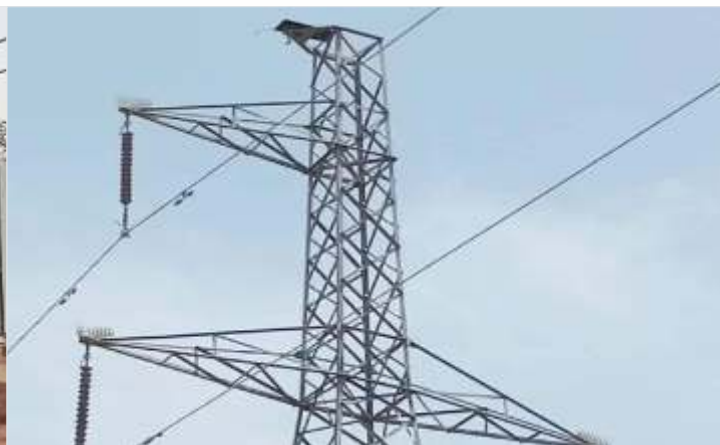
Energized 132kV Shiroro - Tegna - Kotangora Transmission line
