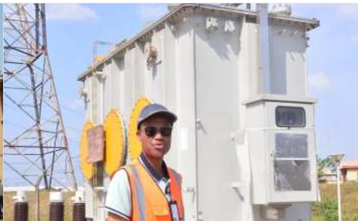
75MX 330kV Shunt Reactor at 330/132/33kV Osogbo Transmission Substation
