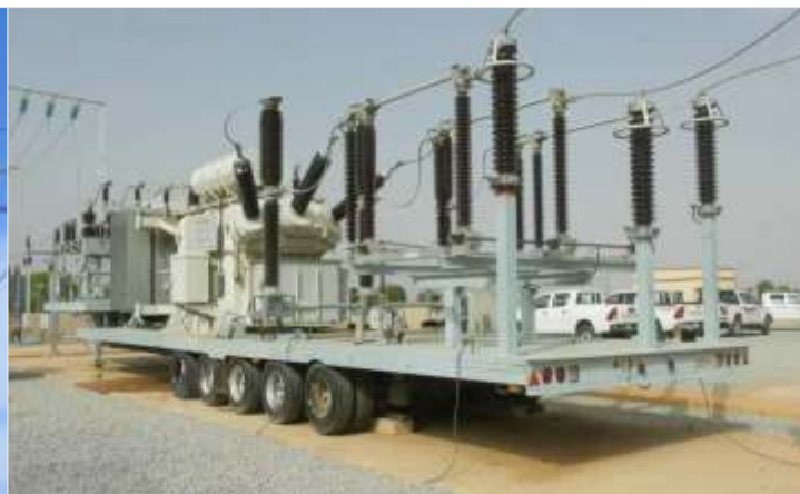
30MVA 132/33kV Mobile Transmission Substation, Bichi
