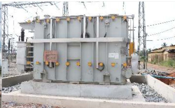
100MVA transformer in Benin Transmission Substation.
